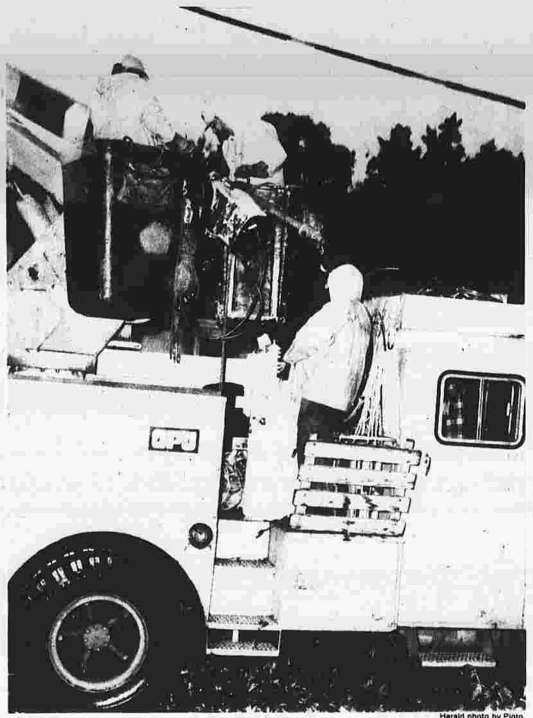
A crew from the Pennsylvania Electric Co. of Johnston, Pa., works on poles and power lines along Crestwood Drive in Manchester Thursday evening despite the falling rain. Northeast Utilities — which brought in crews from outside the state — has come in for criticism from what townspeople and officials say is poor progress in clearing up the damage done last Friday by Hurricane Gloria. But officials said today the state of emergency declared after the storm has been lifted.
